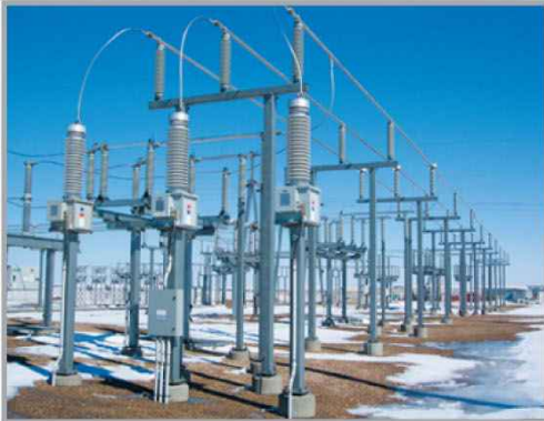
Transmission & Distribution Substations
